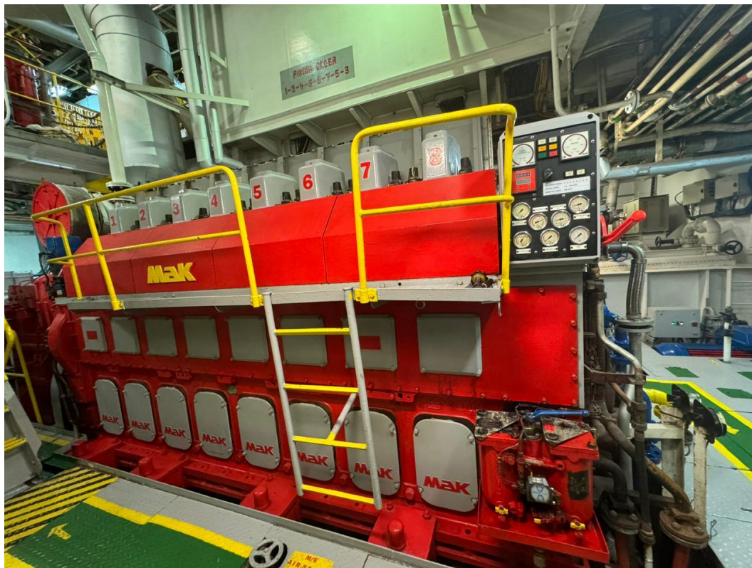
Lampiran 5 : Main Engine MT. VACAMONTE
