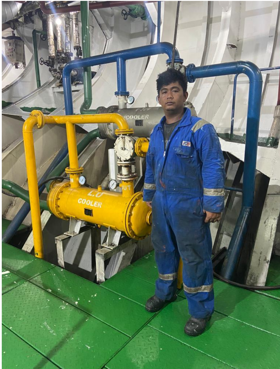
Sumber : Engine Room Mv.Landseador 16
