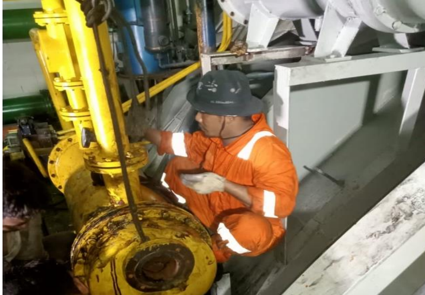
Sumber: Sumber engine control room mv landseador 16
