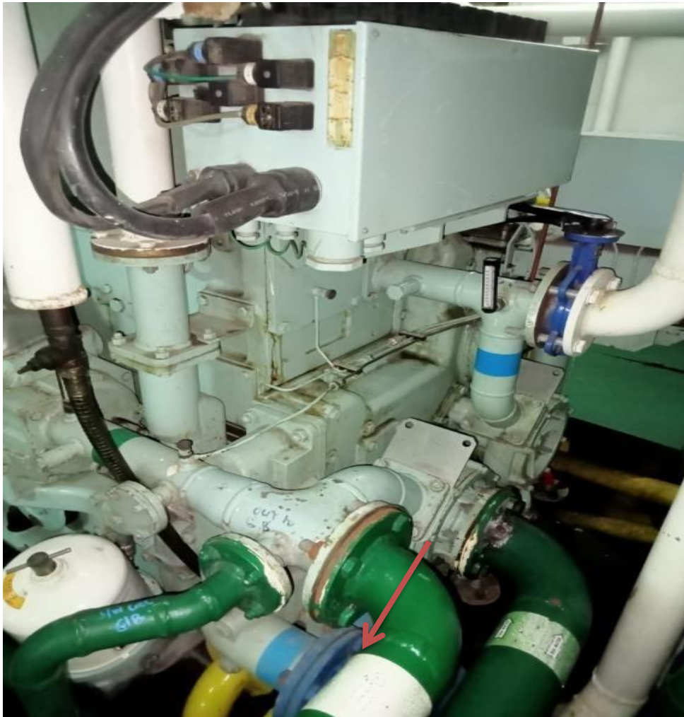
Lampiran 3. Pipa Menuju Main Engine
