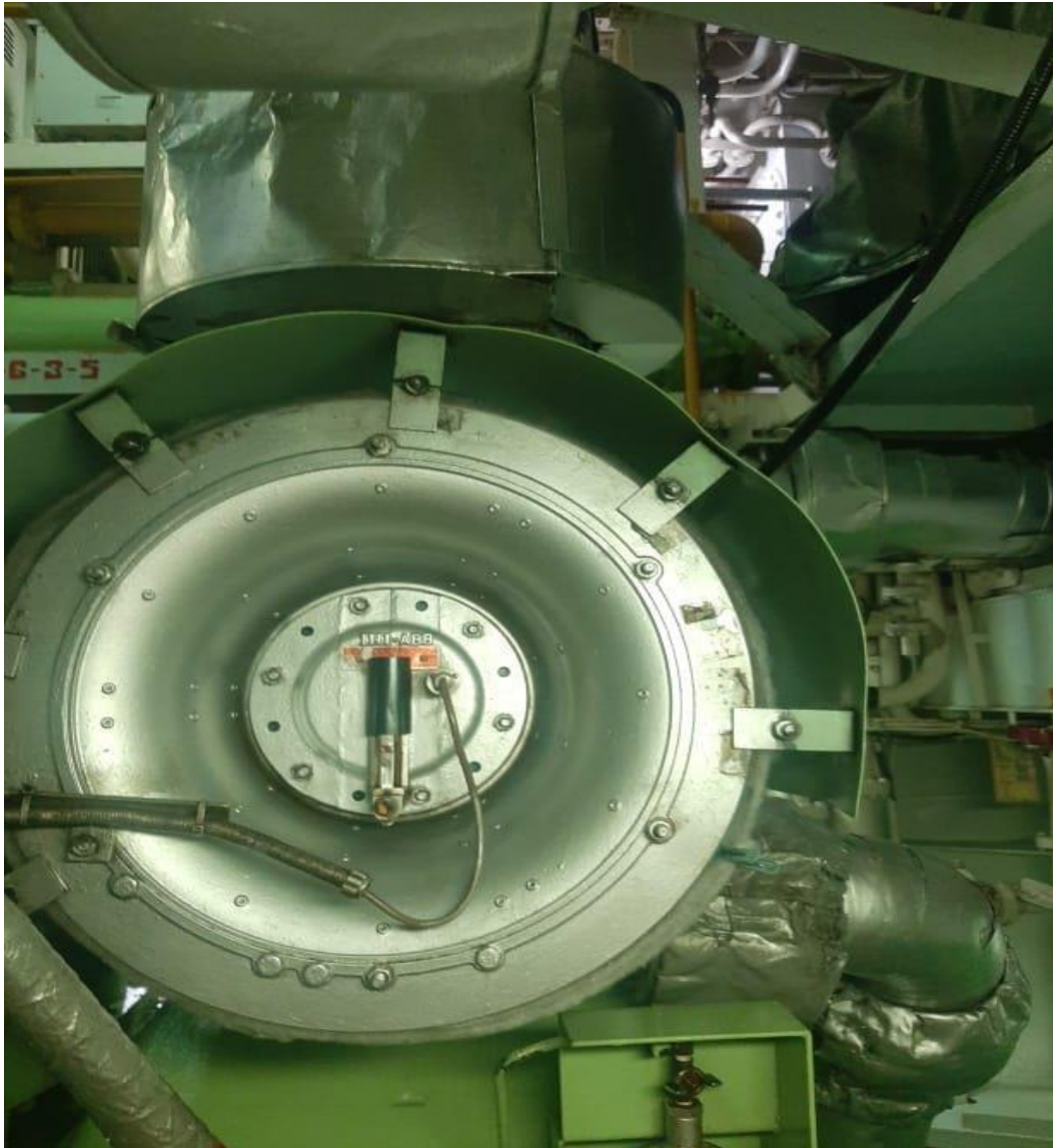
Gambar 7 : Cover Turbin Side
