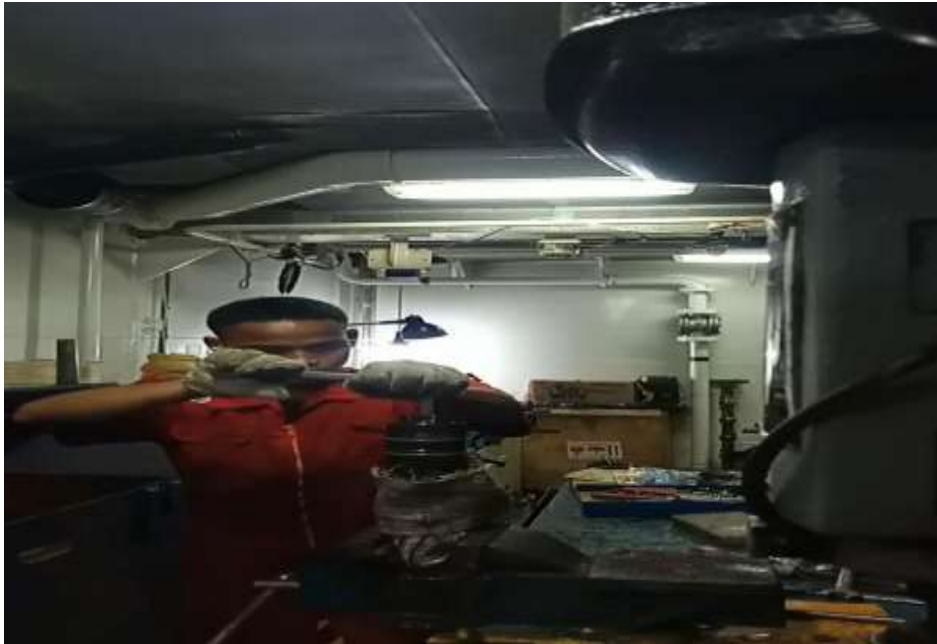
Sumber : Engine Room AHTS.TEMASEK SEPINGGAN
