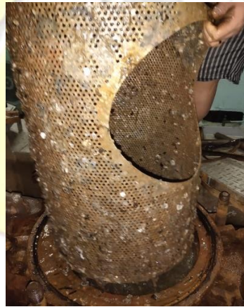
Gambar.1 Filter seach pompa pendingin air laut
