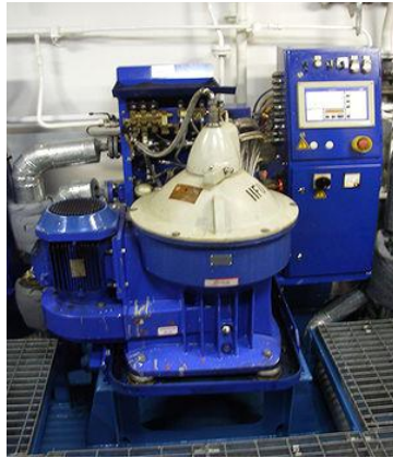
Gambar 2.1. Fresh water generator
