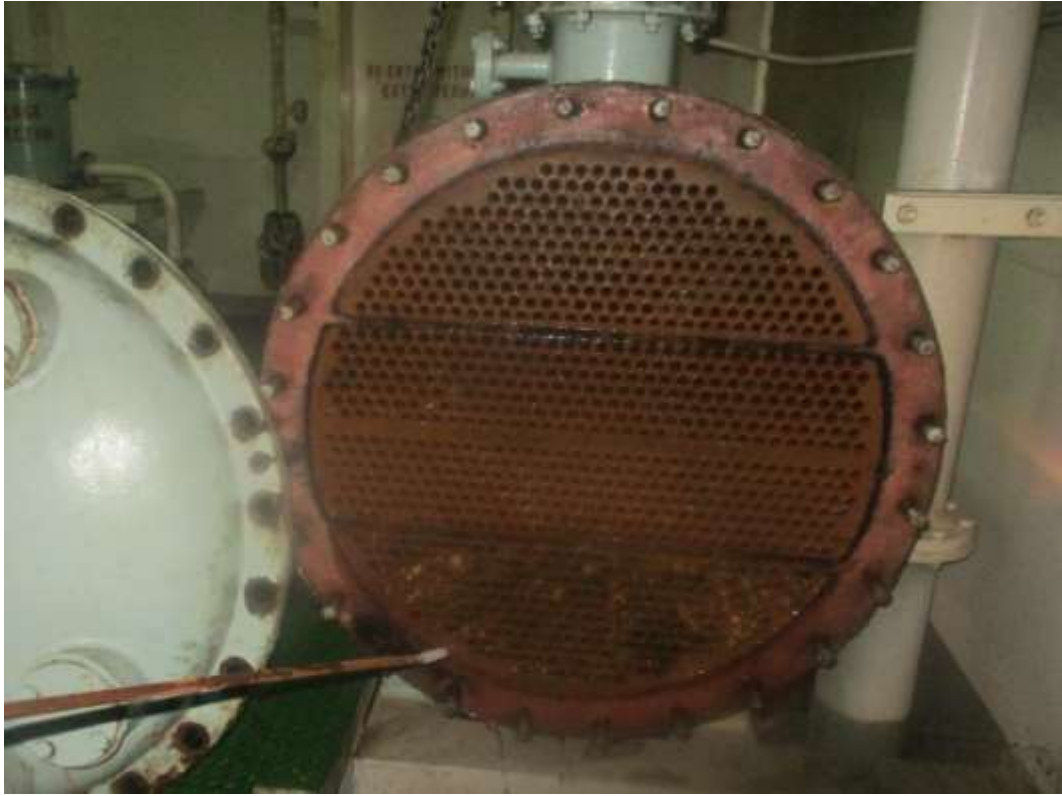
Gambar : Fresh Water Cooler Main Engine Sumber : KM. Dharma Kartika IX, 2021
