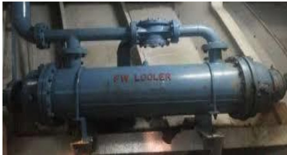
Gambar 2. 5 Fresh Water Cooler
