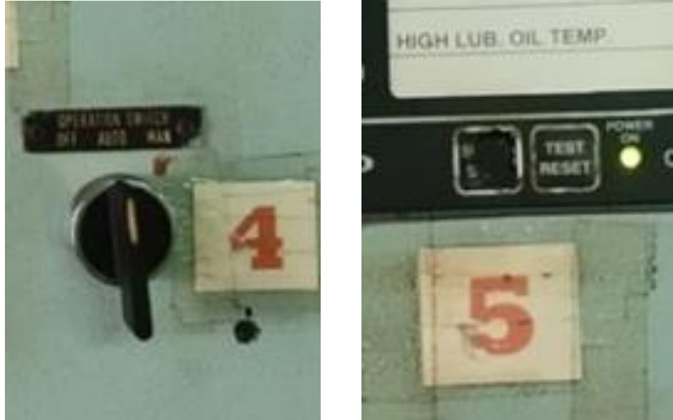
Lampiran 12: Prosedur Pengoprasian emergency generator
