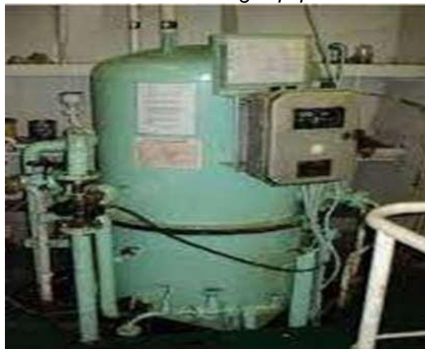
Gambar 2. 6 Oil Filtering Equipment
