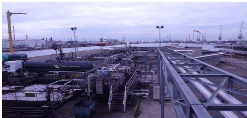
Gambar 2. 10 Port Reception Facilities
