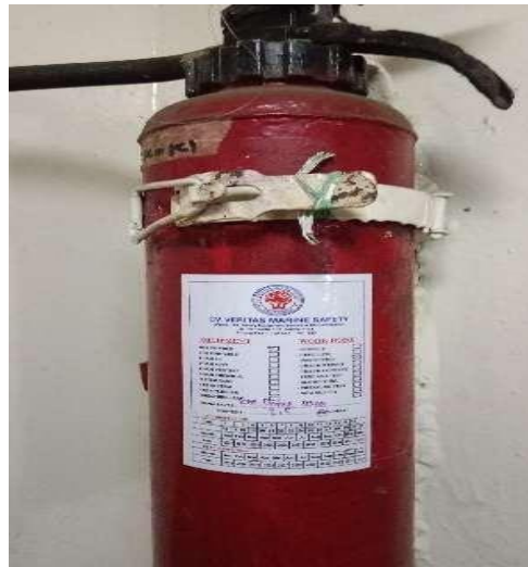
Gambar 2. 2 Fire Extinguisher Tipe Dry powder
