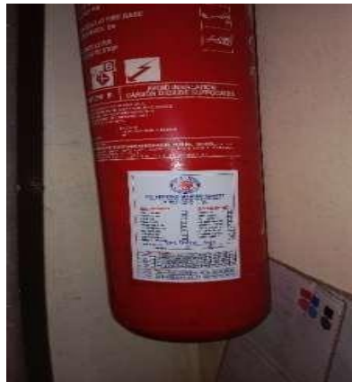
Gambar 2. 4 Fire Extinguisher Tipe CO 2 portable)
