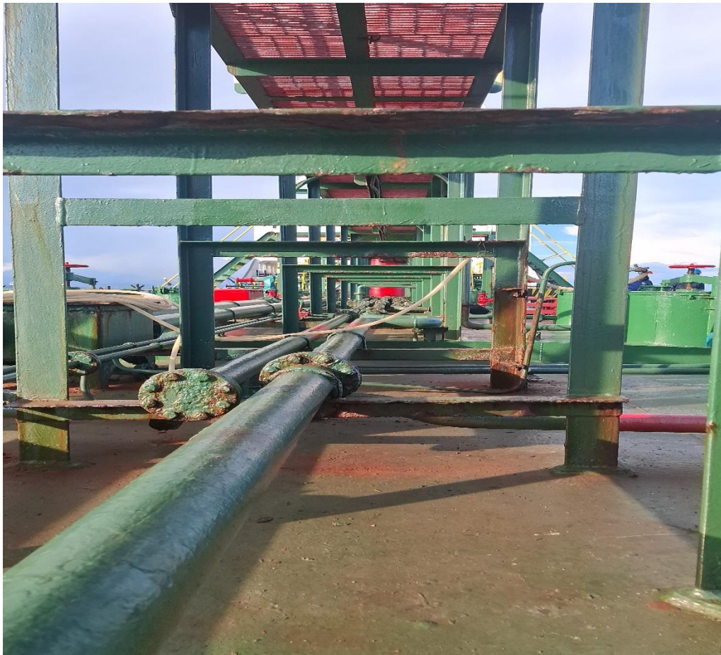
Gambar 2.9 Pipe on deck
