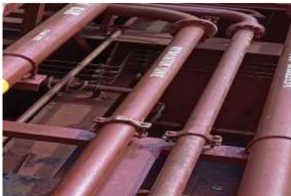
Gambar 2.12 Pipa hydraulic line
