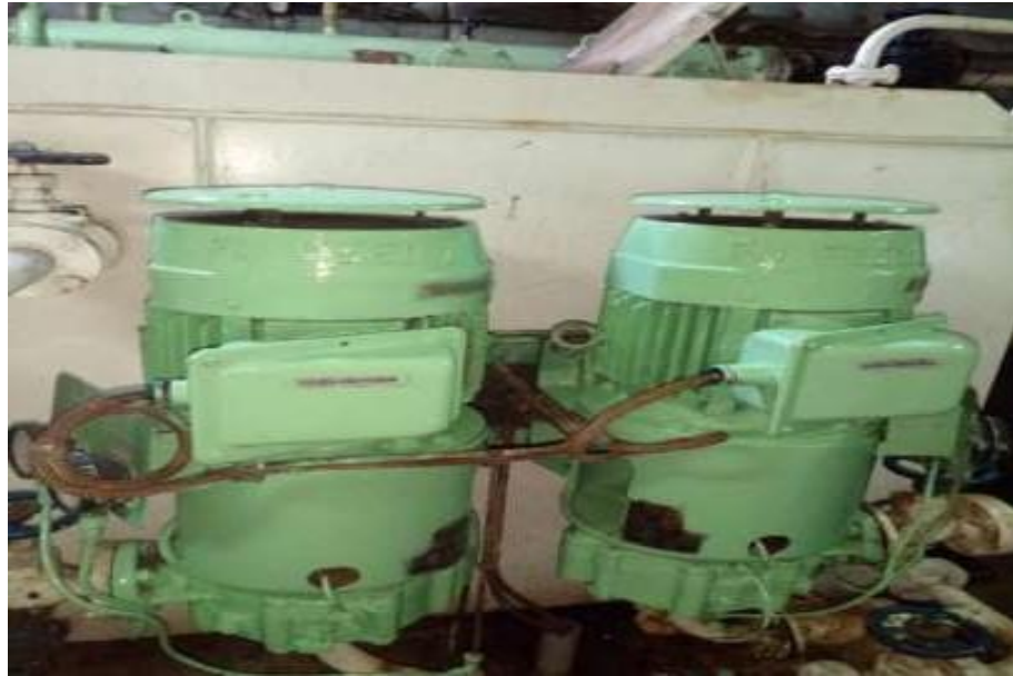
Gambar 2. 13 Feed Water Pump
