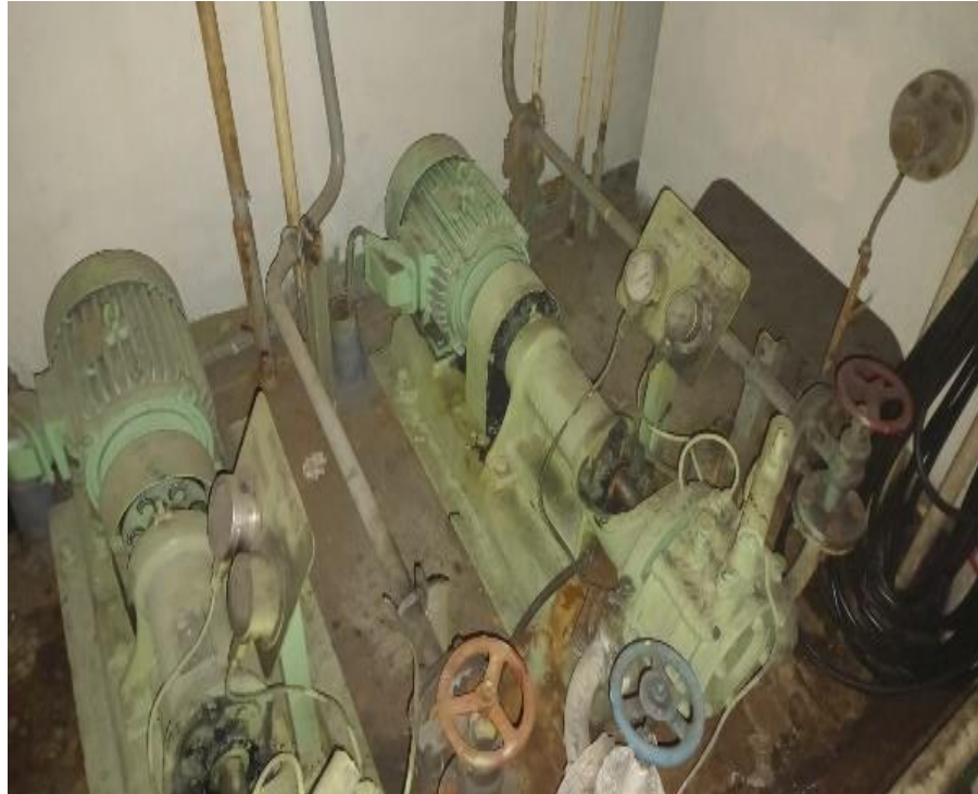
Gambar 2. 8 Feed Water Pump
