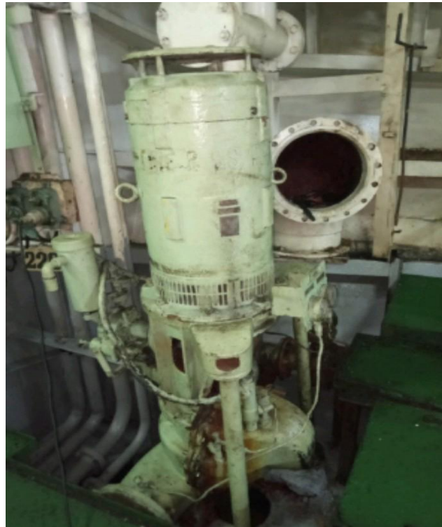
Gambar 2. 1 General Service Pump sumber Mv.LumosoPermai
