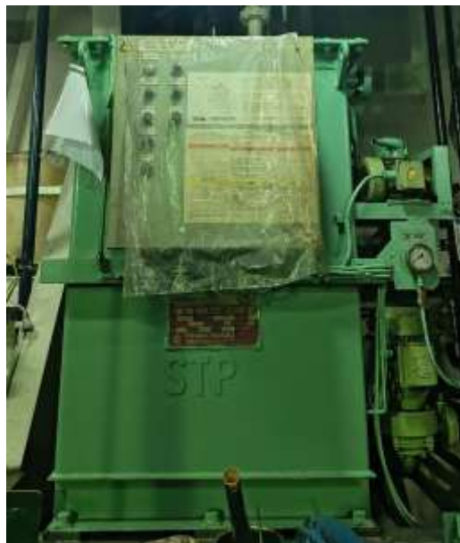
Gambar 2.3 Sewage treatment plant
