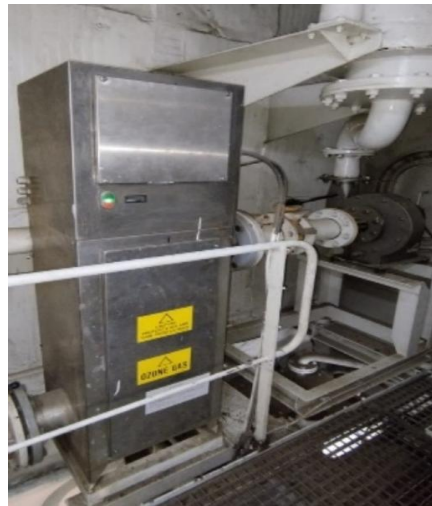
Gambar 2.18 Odour Removal Unit (UV) & Blower
