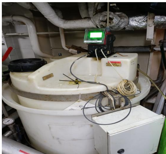
Gambar 2.10 Coagulant Dosing Unit .
