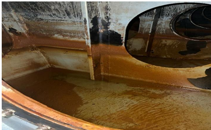
Gambar 2.17 Treated water Holding Tank
