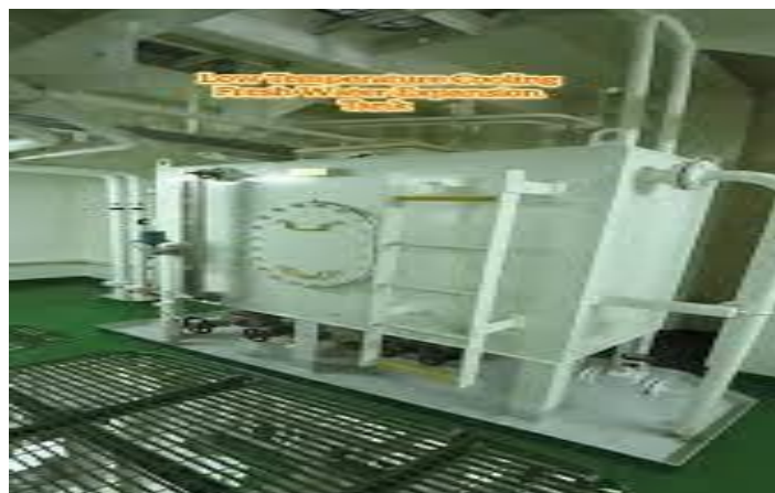
Gambar 2. 4 Fresh water Expansion Tank
