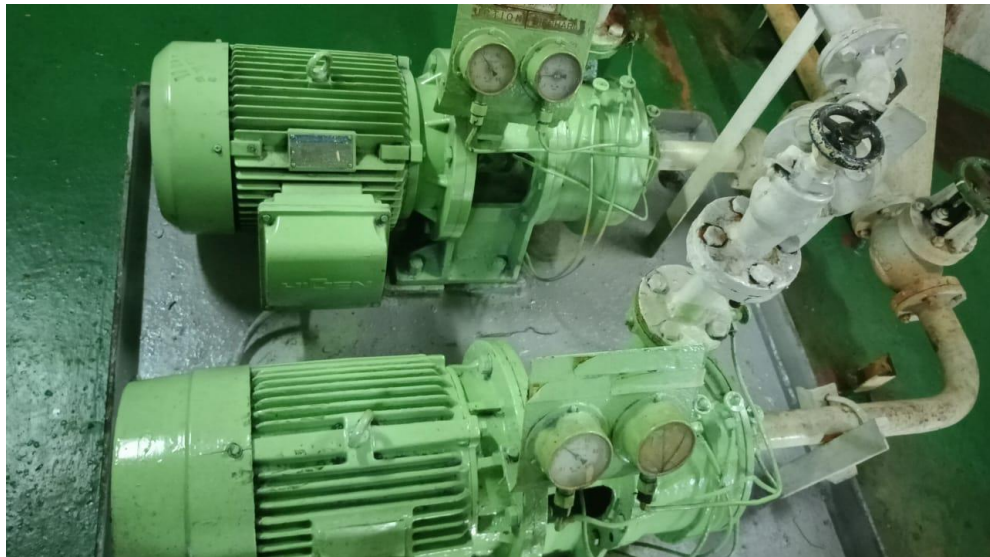
Gambar 2. 8 Feed Water Pump
