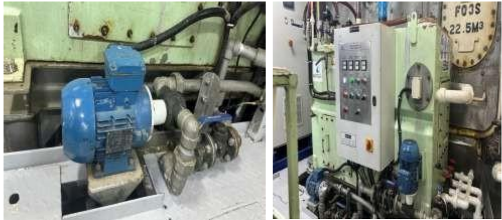
Gambar 8. Discharge pump and Piping
