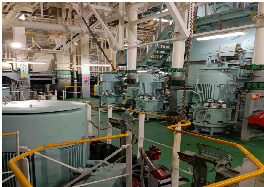
Gambar 2.8 : Sea water supply pump
