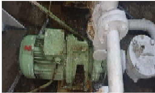
Gambar. 2.9 Cooling water circulating pump
