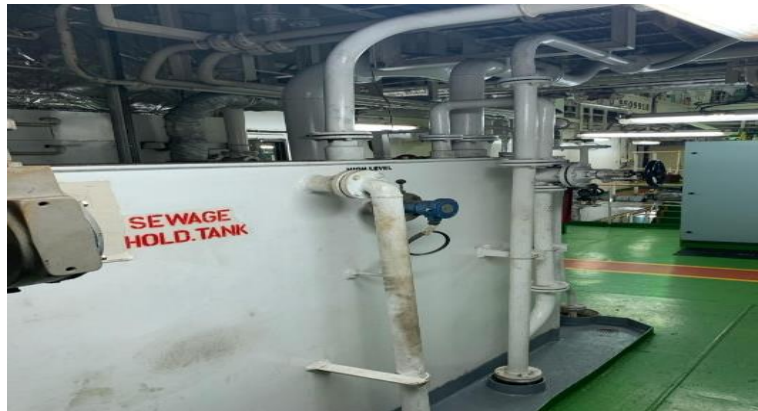
Gambar 2. 8 Sewage Holding Tank.
